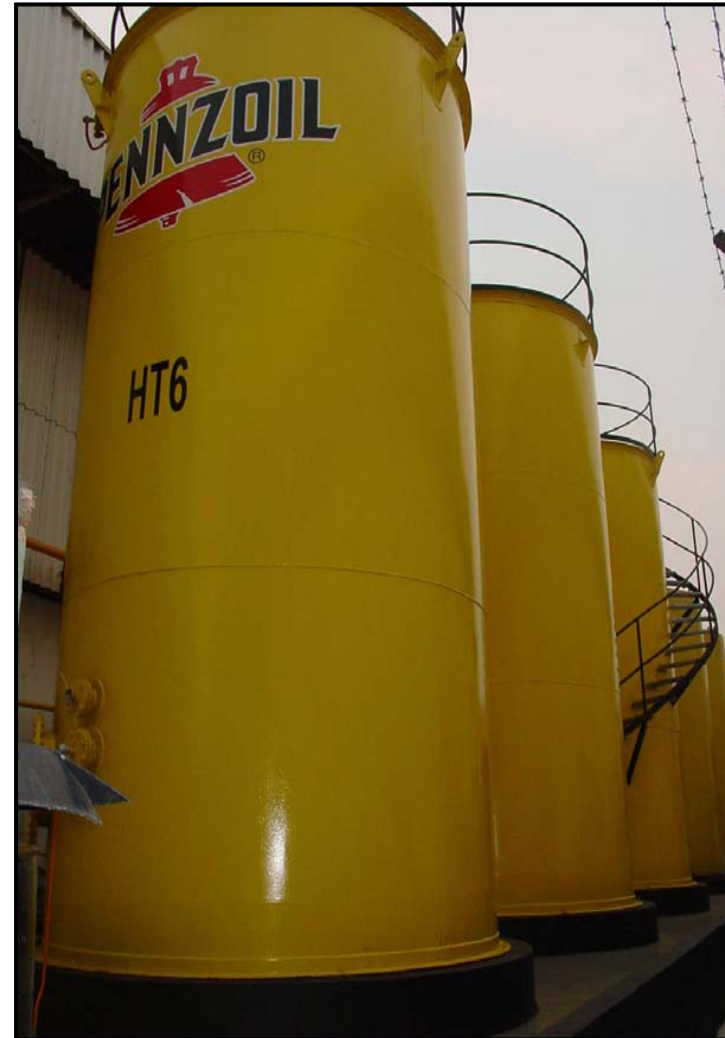
Oil Storage Tanks
